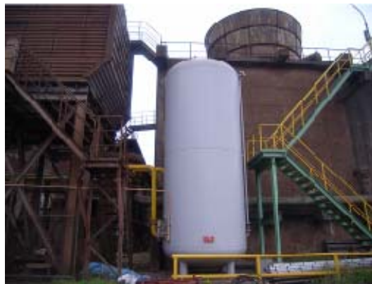
Photo 4 – COG Receiver Tank
