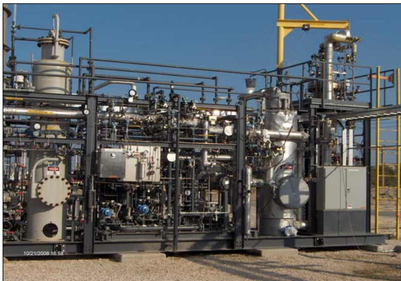
Figure 7: RGP Pilot Unit at a US Refinery
